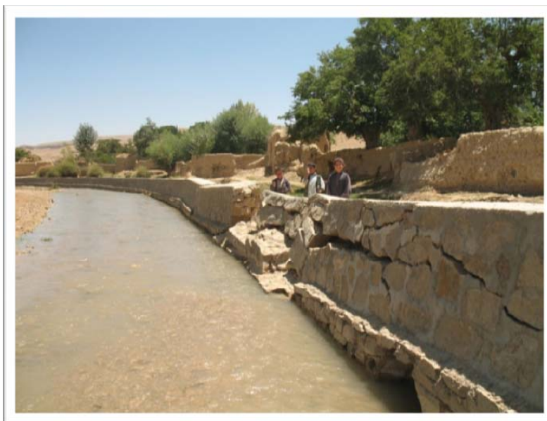
Illustration 5: Sayghan District, Bamyan CDC-constructed retaining wall that has collapsed
